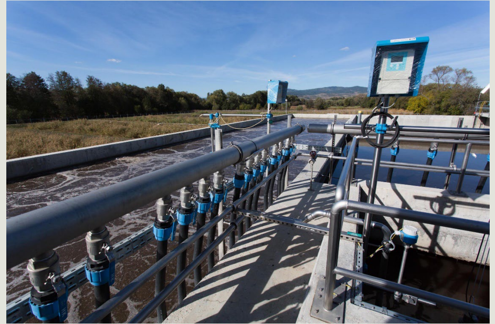
WWTP Berovo – Capacity 14'000 citizens
