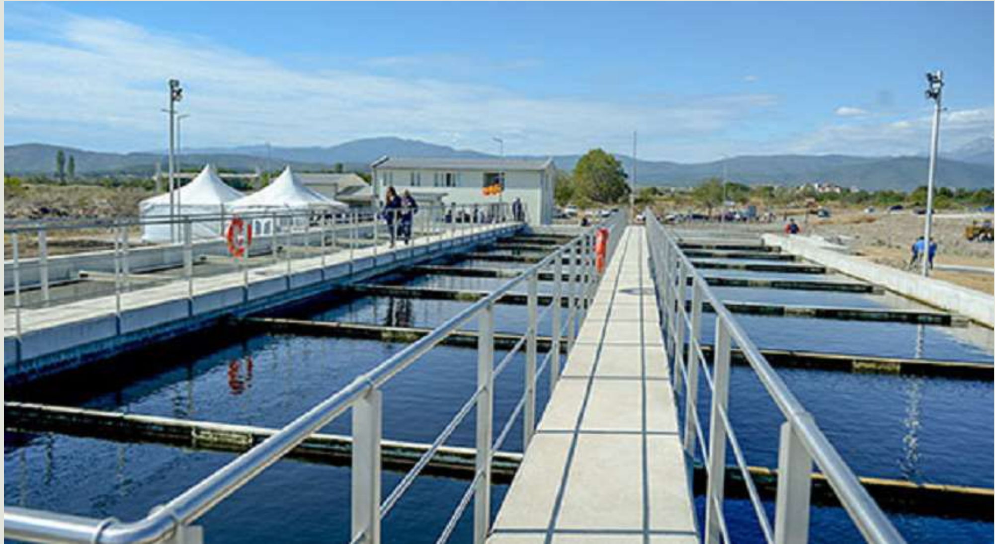
WWTP Gevgelija – Capacity 16'000 citizens
